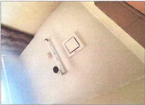
EXISTING CEILING AND LIGHTINGS NOTE: NEED REPAINTING AND INSTALL NEW LIGHTING
