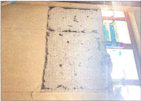
EXISTING WALL TILE NOTE: CHIP OFF AND REMOVE ALL CRACKED EXISTING WALL TILES.
